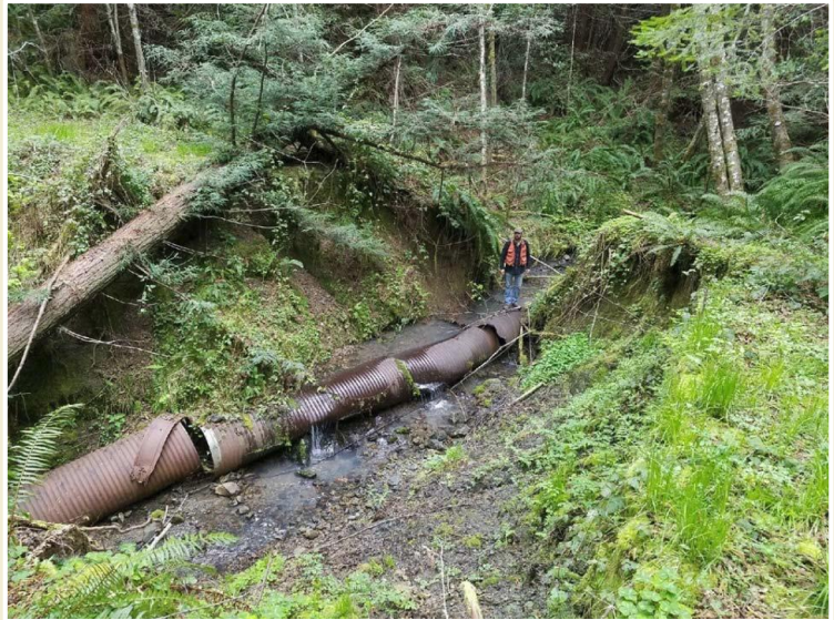
A washed out culverted stream crossing (Feature #322) within the Cañon Creek Assessment Area. Credit: PWA.
